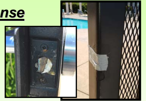
Gate latch found disabled during routine inspection
