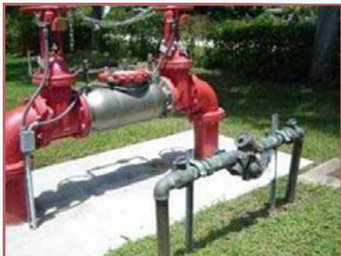
Cross Connection device
